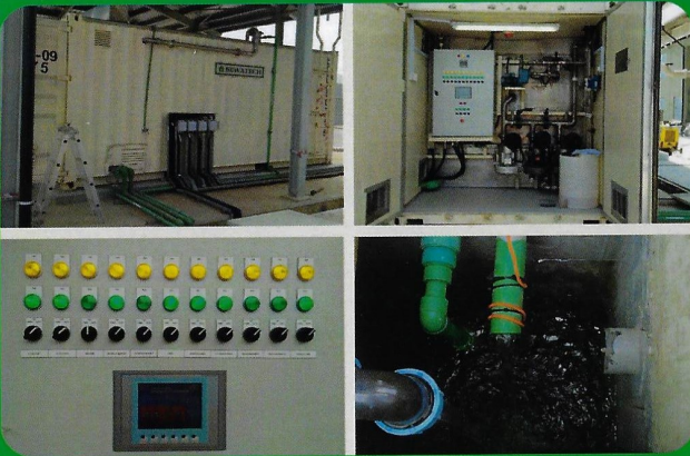
STP FOR TOTAL E&P NIGERIA AT OBAGI
