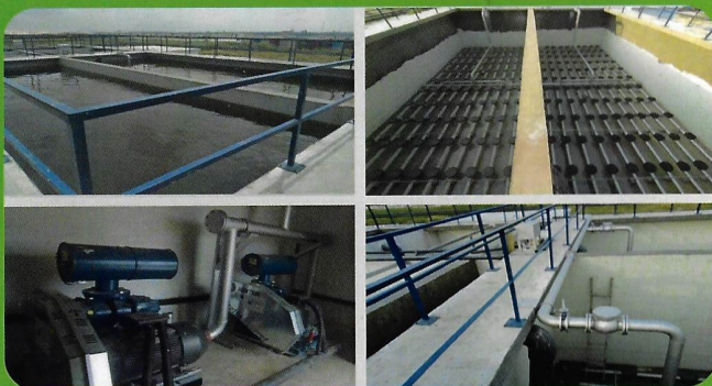
STP FOR REFINERY
