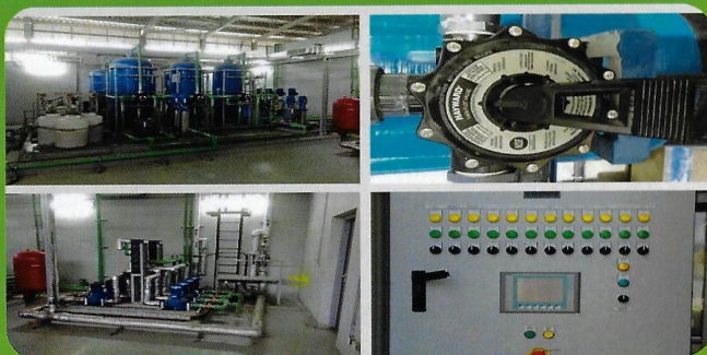
STP FOR TOTAL E&P NIGERIA AT OBAGI
